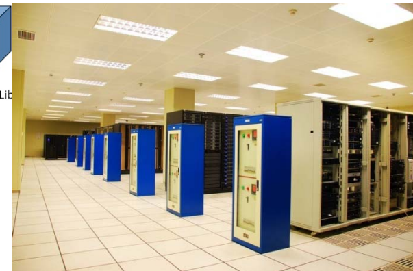
Power supply & cooling system
