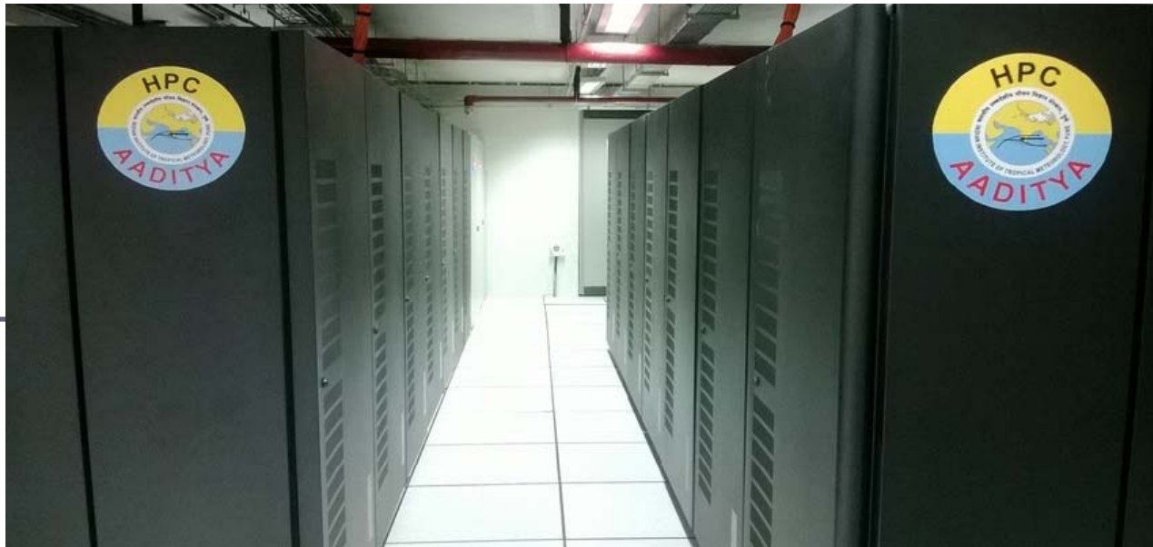
IITM's HPC Facility - AADITYA (790+TF system)
