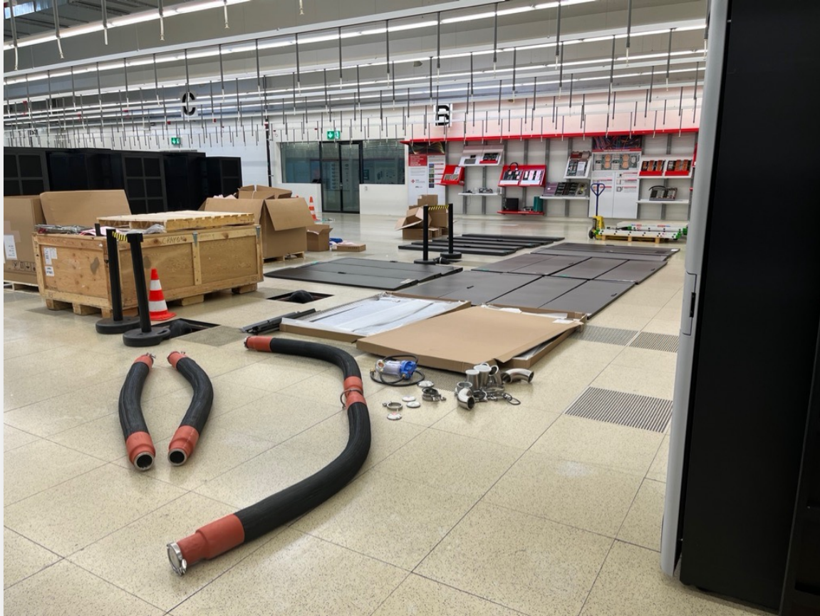
internal pipes, doors and panels
