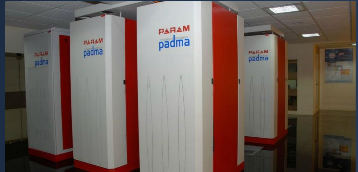
PARAM Padma @ CDAC, Bangalore First supercomputer in Top500.org
