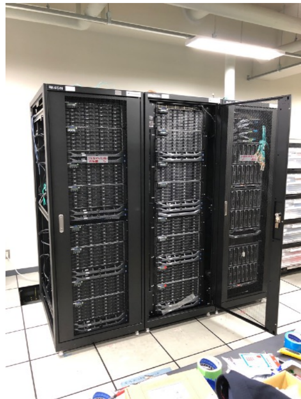
Reduced system (3 server racks)
